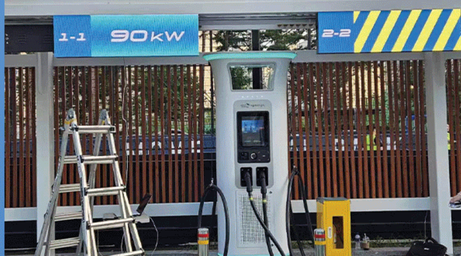
Korea Charging Station Project
